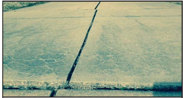
ASR Cracking and Expansion in Sidewalk
