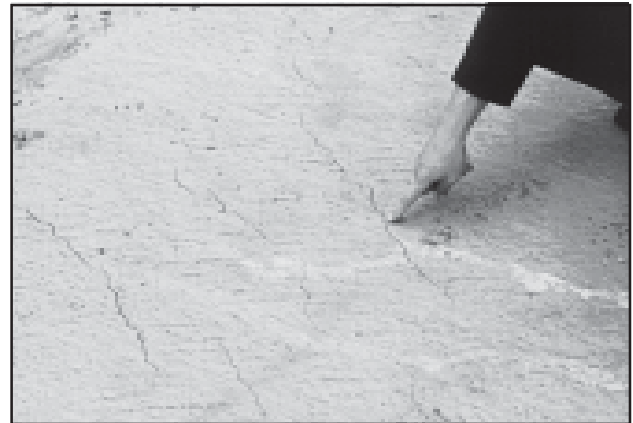
Plastic Shrinkage Cracks
